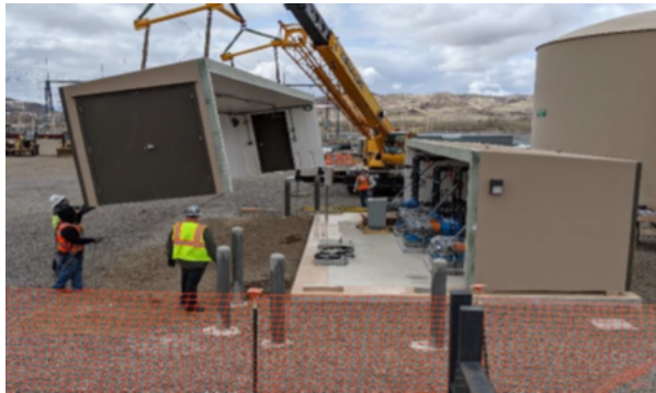
Figure 2. Vertiport landing pad, mini data center, infused FRP building
