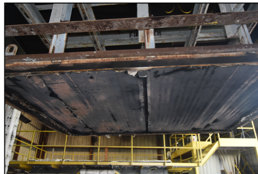
Underside of panel removed from furnace
