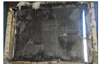
Panel after fire hose spray
