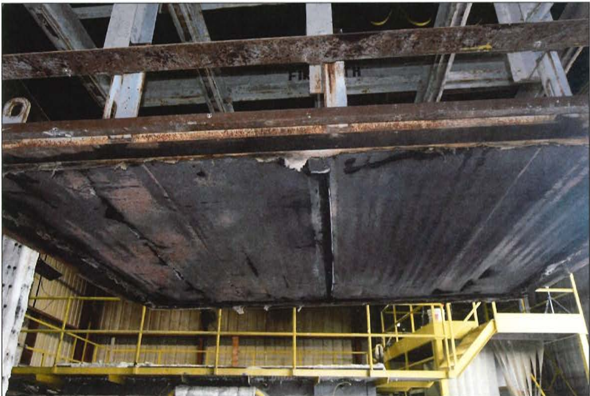
Figure C-12. Exposed Side of Serial No. 4001a Floor Assembly after Cooling.
