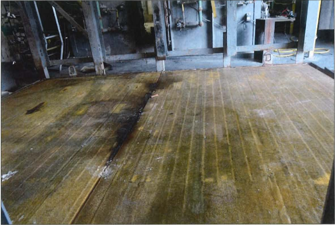
Figure C-11. Unexposed Side of Serial No. 4001a Floor Assembly after Removal of Jacks.
