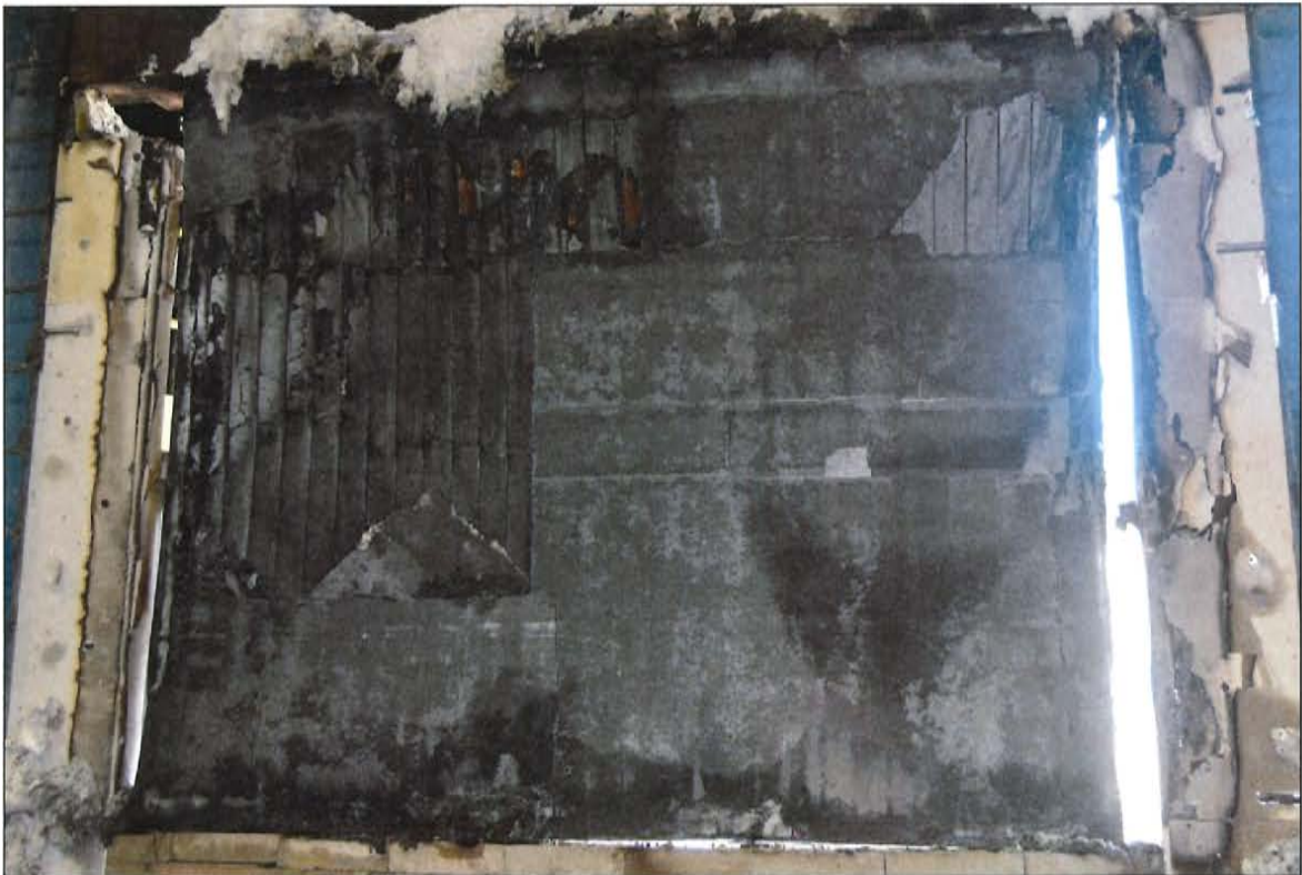
Figure C-12. Exposed Side of Serial No. 4001b Wall Assembly after Hose Stream Test.
