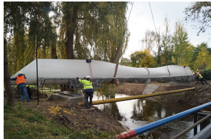
Below: Construction workers install a footbridge across the Szprotawa River in Poland. Photo from Anmet
