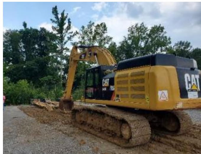
Figure 30. 110,000 lb CAT used to conduct the proof testing. There is sludge and wet soil due to heavy rains before the tests.
