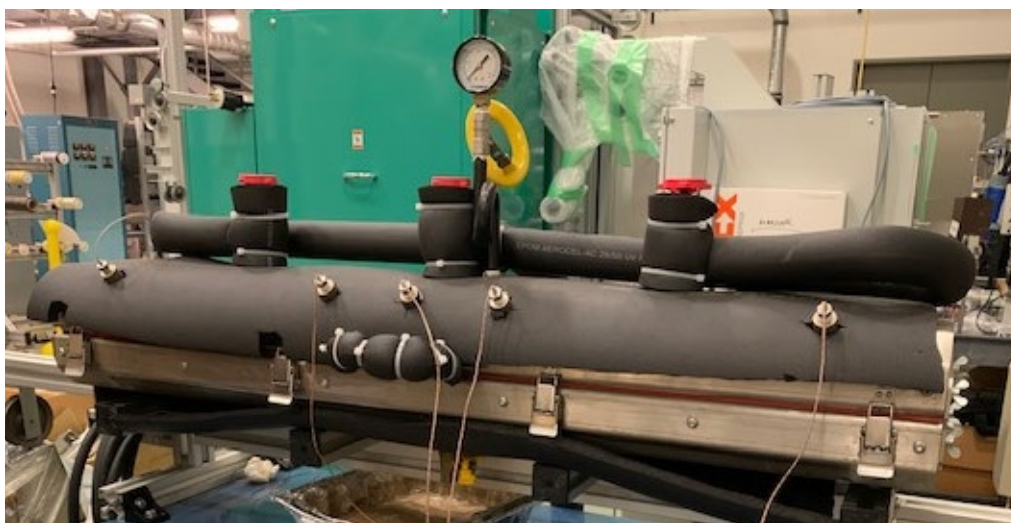
Figure 3 ORNL Steam Stretcher
