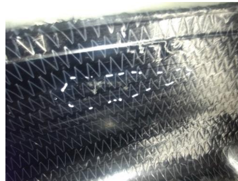
Region with defects
